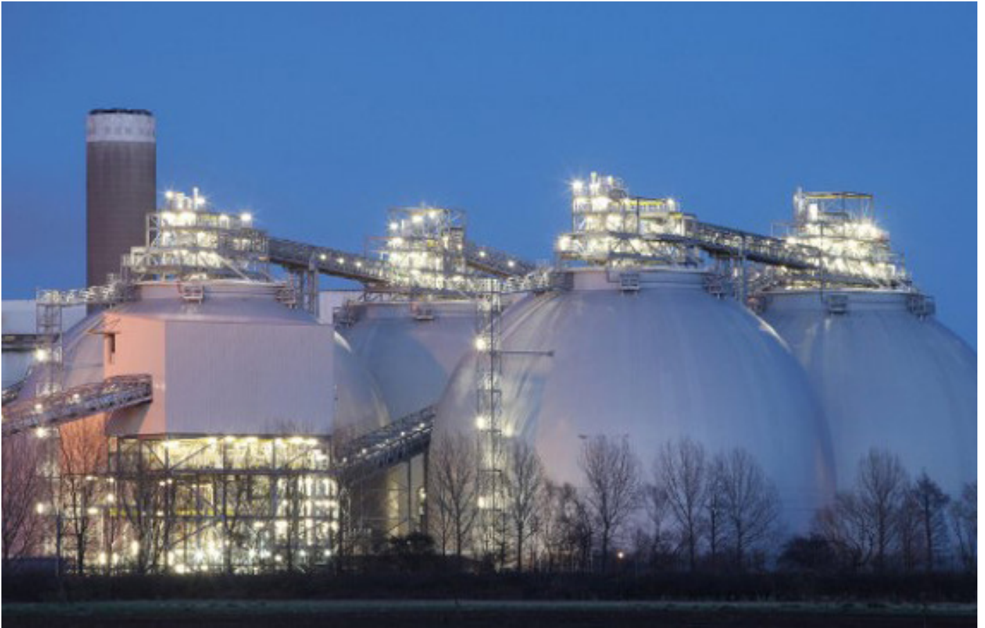
Biomass domes at Drax Power Station, Yorkshire, on which Bioenergy Carbon Capture and Storage (BECCS) technologies are being piloted (Drax)
